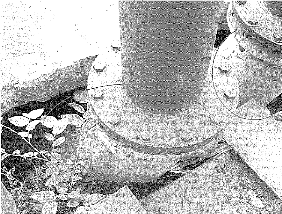
Pic 03: Others ash pipes and bends Under ground
